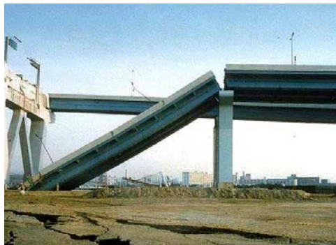
Failed bridge, earthquake of 6.8 magnitude Kobe, Japan 1995
