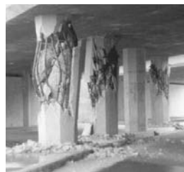
Damage resulting from the Magnitude 6.6 earthquake, San Fernando Valley, California.
