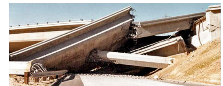
Highway collapse, earthquake of 6.6 magnitude, San Fernando, CA 1971
