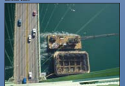
A bird's eye view. Only birds and airplane pilots enjoy this view of the Narrows Bridge, new caisson and work barges. Around the clock support from the marine and land side was necessary to build the caissons that reached the seabed floor in December 2003 (Gig Harbor) and January 2004 (Tacoma). Fall 2003
