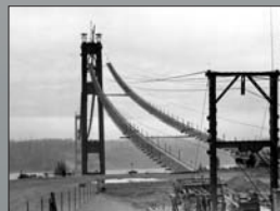
The making of suspension cables. Temporary catwalks were placed from tower to tower, allowing crews to work on the cables. The bridge's two suspension cables were spun from wire spools. The wire was unreeled on site and affixed to an anchorage built on land at each end.
