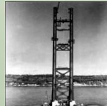
Raising up the new towers. Crews used a "crawler crane" to build the towers. Laborers worked six months to complete each tower leg. The legs of the 1950 towers are made of hollow steel cells, stacked on top of one another. The cell sections are four columns arranged to form a hollow cone in the center. Each section is 30 feet long and weighs 27 tons. To stabilize the towers during construction, temporary "outriggers" were added until the cables and deck trusses were completed.
