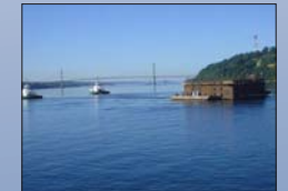
From shipyard to port. Massive barge gently coasts a gentle part of a caisson from the Port of Tacoma to its final resting place just south of the existing bridge. Above the water line can be seen corrugated steel panels, which are the caisson's "steel skin," providing a watertight environment for placing concrete in the dry. Favorable tides, knowledgeable mariners and a tremendous amount of planning contributed to a smooth and successful voyage. Summer 2003
