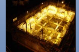
Night fall, crews kept on. Lights illuminating the caisson at night allowed crews to keep up an aggressive construction schedule almost around the clock. Summer 2003
