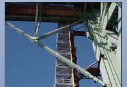
Getting to "Pier Top City." Convenient access to the caisson construction site is provided by this temporary 21-story stairway. Supported by the existing bridge's tower, it descends to "Pier Top City," the nickname for temporary offices placed on the existing bridge caisson. Spring 2003
