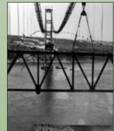
Raising a deck. The deck of the second bridge was built quite differently than the deck of the first. Crews raised steel beams singly or in sections. Assembling the deck, piece by piece, was like assembling a giant triceratops.
