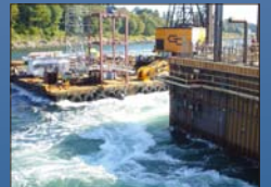
Bridge-building in swift currents. The apparent whitewater rapids shown here are actually water churning from tidal currents in the Narrows channel. During the construction of the caissons, the currents reached 20 to 24 knots, creating unique marine challenges to the designers and builders. Spring 2003
