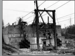
Anchorage construction. This anchorage and its twin on the opposite shore of the Narrows supported the bridge and traffic using it. The concept is being used today.
