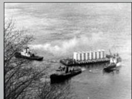
Caisson in tow. Here, the first section of the lower foundation, the hollow caisson, was towed into place. It was secured to anchors that had previously been placed on the seabed. Creating the lower foundation was a gradual process of repetitively building layers of steel and concrete. Slowly, the pier "grew" upward as it sank downward toward the seabed.
