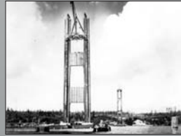
Standing like sentries in the Narrows. Towers were built on top of each pier pedestal and finished with a steel saddle on its highest point. The saddle of each tower is where the main suspension cable is secured.
