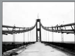
Building the Deck. For the first bridge, the deck was constructed with pre-formed steel sections. This section was carried to the bridge on scows, lifted up and attached to the cables. When all the steel sections were tacked into place, the deck was ready to receive its concrete surface.
