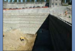
A man-made canyon. The eastern (Tacoma) anchorage was built into a site excavated almost 65 feet deep. The main standing at the top right of the photo is shored by the hole that was filled with reinforced concrete shortly thereafter. Summer 2003
