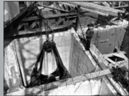
Dredging the Narrows. As a result of dredging the seabed, the caisson's steel cutting edge met and sank into the earth. The pier was then excavated to the proper depth through its hollow cone (dredge wells).
