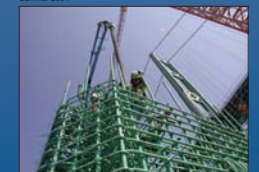
Birth of a tower. With the 1950 bridge's towers in the background, a female worker focuses on the task at hand — pouring the first concrete of the new towers. Reinforced with layers of precast steel rebar, the concrete towers will rise 510 feet into the sky to stand tall and ready to their more massive bridge companions. Summer 2004
