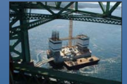
Working on water. The white structures, or "brackets," sitting on each Gig Harbor tower leg house the concrete forms that crews use to place concrete as the towers rise. Jutting from the top of the forms is steel rebar that reinforces the lower concrete. A refractable walkway (lower left) provides construction access to the towers from the existing bridge. Summer 2004
