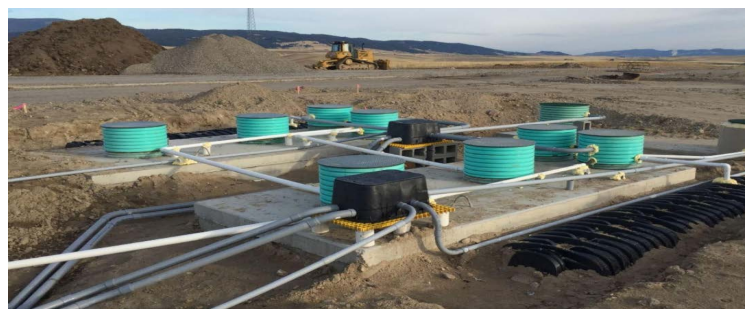
Montana safety rest areas wastewater treatment, Source: CDM Smith Contracting
